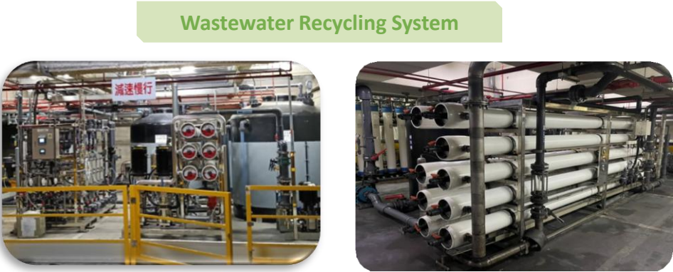
The grinding wastewater recycling system treats and reuses wastewater, improving water-use efficiency and promoting circular water resource management.
